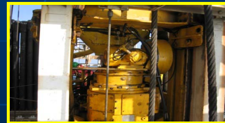
Check Blower Housing is Secure
